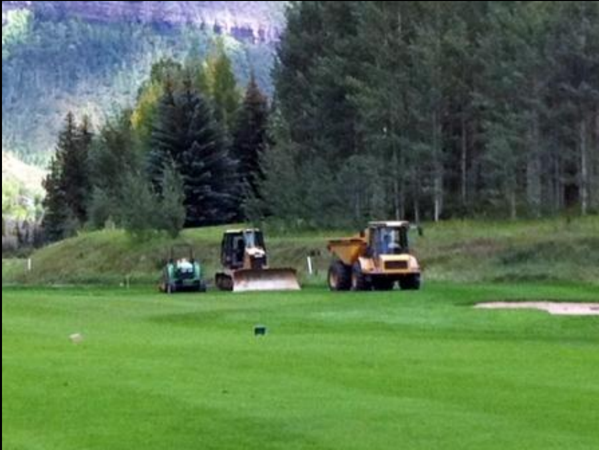
Town of Vail Construction begins on the relocation and downsizing of the 18th Green. (photo by property owner)
