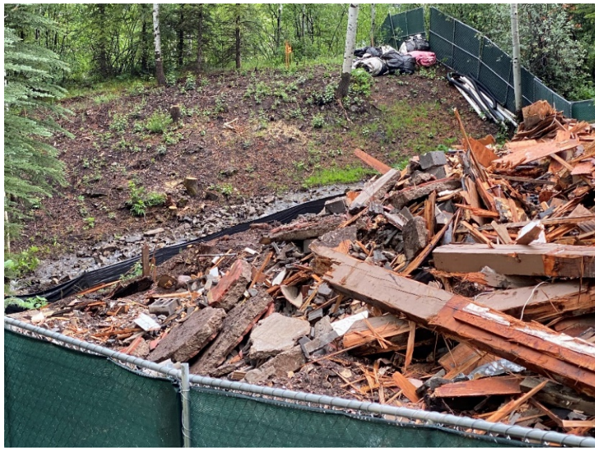
Rockledge Road demo/rebuild with site cleared of much of its vegetation and its stream channelized.
