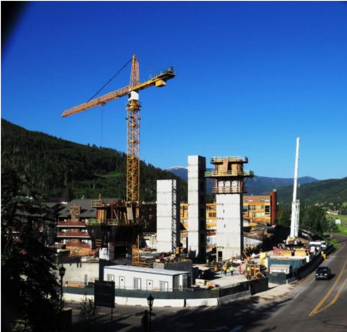
The Vail Lion Building Under Construction: Shown Are Parking Levels and Elevator Shafts - Frontage Road Lanes Shown Right
